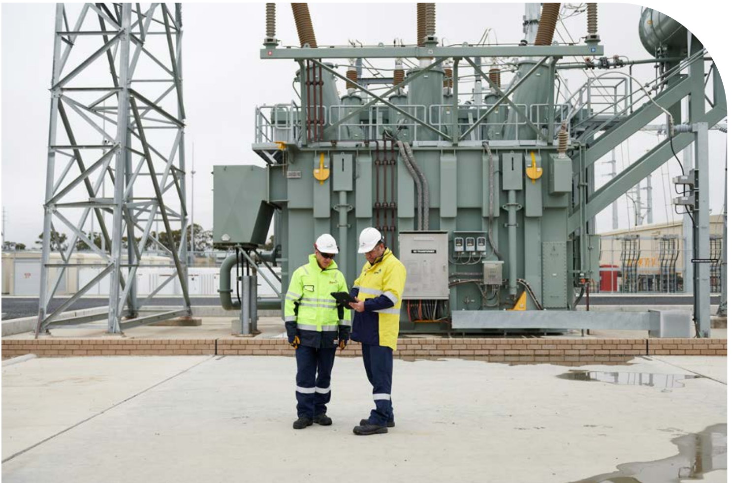
Transformers play an important role at terminal stations.
