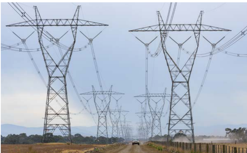
Single circuit transmission towers
